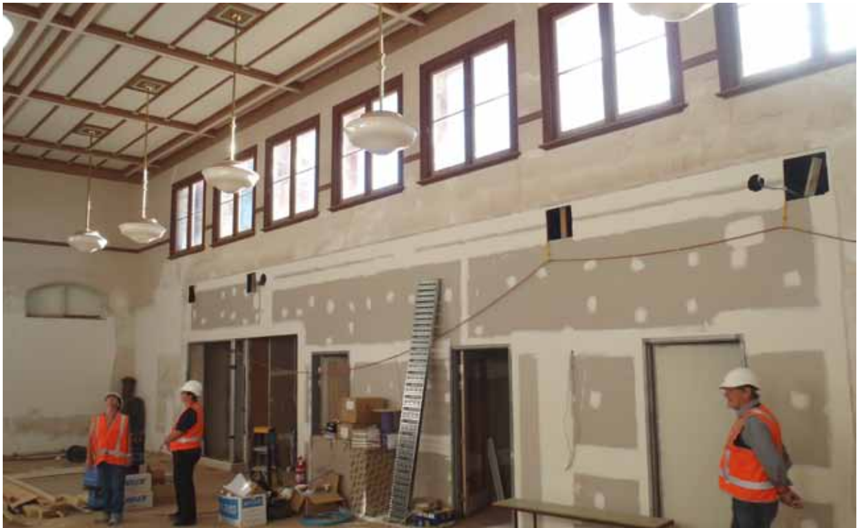
The former main Post Office hall will become the new Registry area at Kalgoorlie Court.
