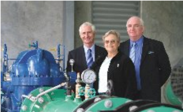
Minister for Water Resources Mr John Kobelke, Board Chairman Mrs Diana Phillips and Chief Executive Officer Brad Bevis at the official opening of the City Waterlink Project.
